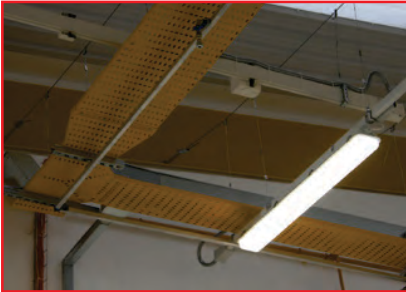
Busbar and Lighting
