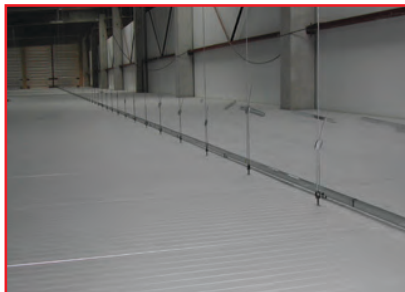
Under panel lighting
