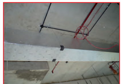
PI foam ducting
