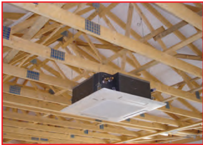
Air conditioning units
