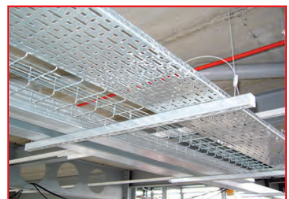
Multiple cable trays on single channel
