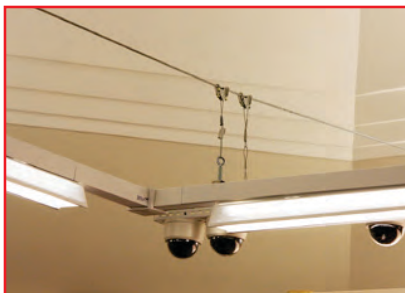
Lighting and Camera on Catenary
